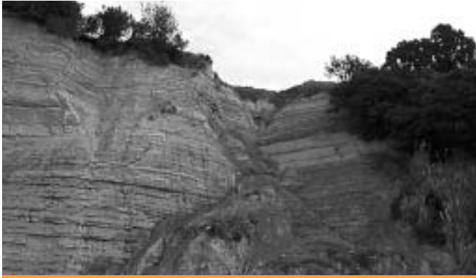
Wedge failure below Takapuna Grammar School that has occurred at the intersection of a fault plane (on right) and a joint (on left).
