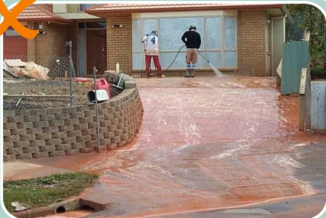
Poor practice - exposing aggregate without any controls
