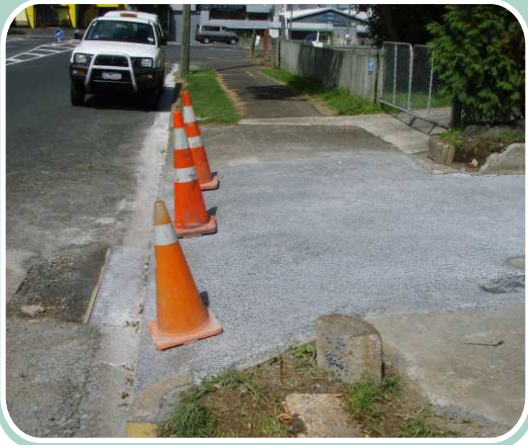
Exposed aggregate driveway undertaken without controls
