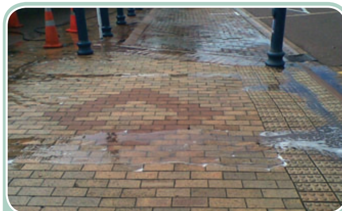
Sidewalk being waterblasted without controls in place
