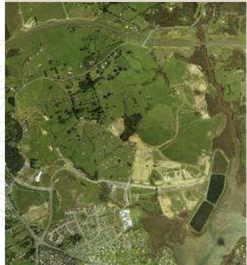
An aerial view of the Silverdale North Precincts 1-7 during construction undertaken by Hick Bros Civil Construction Ltd.
