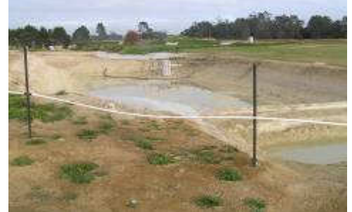
HEB Construction Ltd during construction of the stormwater pond associated with stage 3 & 4 at Hingaia Peninsula.
