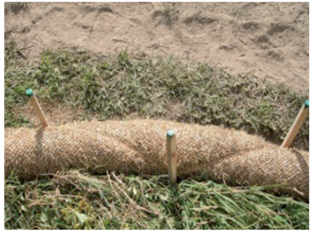
Straw sock secured in place using stakes and bale twine; note that the stakes are placed every 600mm.
