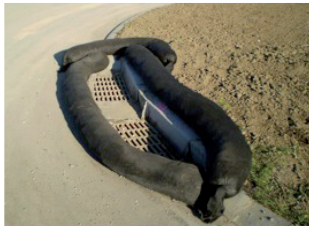
Compost sock used for inlet protection; note the overlap on the up-slope.
