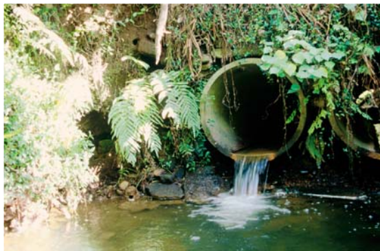
Photo 1: A poorly constructed culvert with overhanging outlet.
