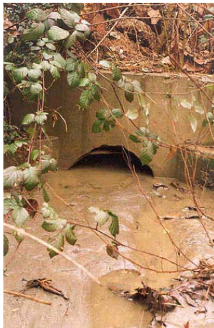
Photo 2: Uncontrolled works resulting in gross sediment discharge into stream.
