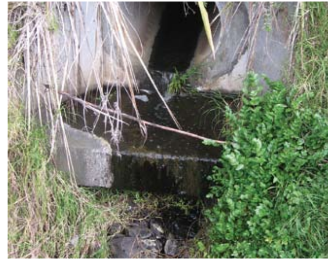
Culvert impassable by native fish.
