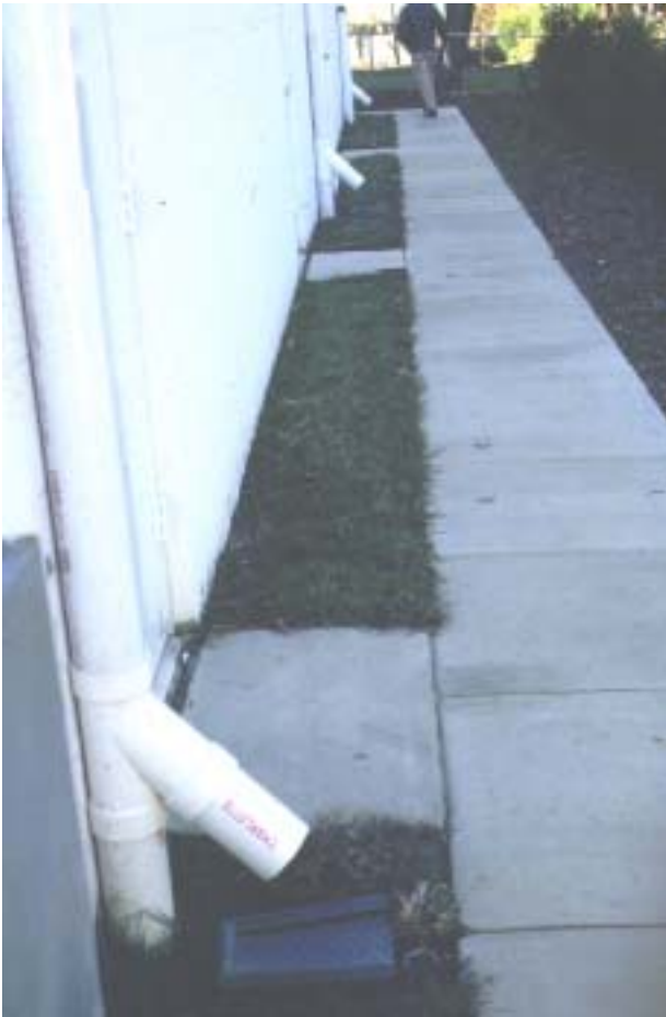
Plate 8-4: Infiltration dry well
